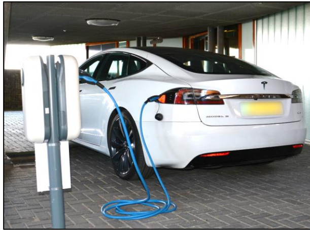
EV-laadpaal parkeergarage Nauerna
